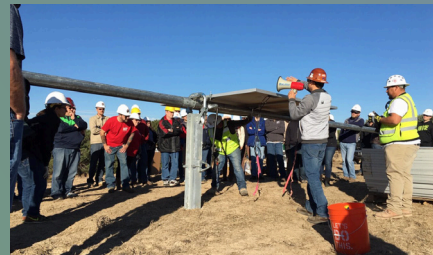
In 2016 CEA helped the Idaho Youth Ranch install a 100 kW PV system, which helped to reduce its annual greenhouse gas emissions by 200 tons.
