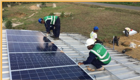
In 2017 CEA designed, procured, and installed a 2.6 kW PV system for an off-grid medical center in Southern Cameroon.
